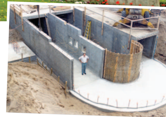
Owner Ken Konrad during the construction of Konrad Marine's 80,000 gallon underground test tank that was completed in 1996.
